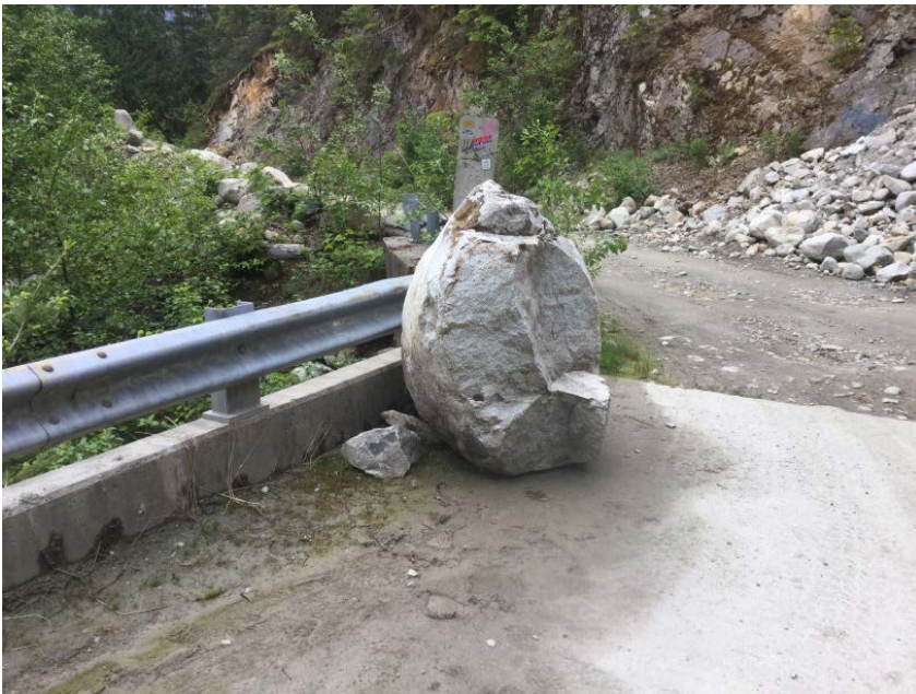
Debris on deck
