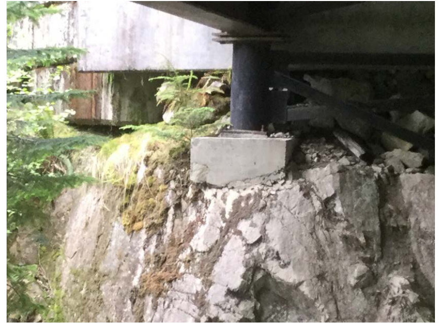
DS right bank footing appears to have spalled and patched in the past
