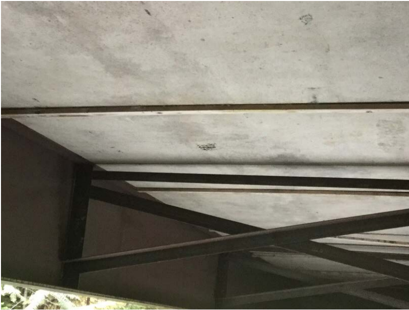
Spall look caged approx centre of span US
