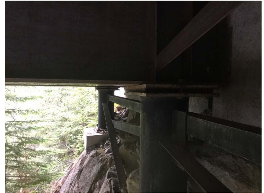
Centre right bank bearing is slightly deformed, typical for 2 other right bank bearings
